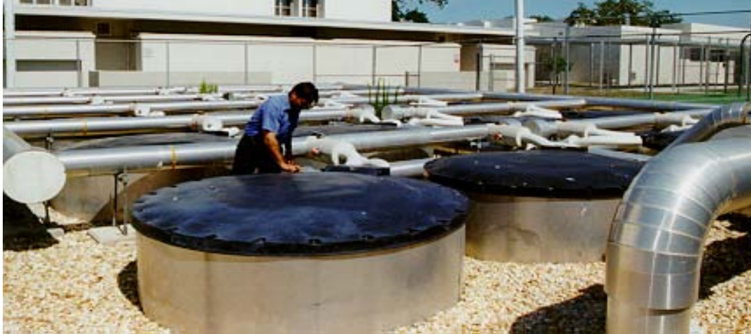
Figure 4.2.3 Ice Storage Units
