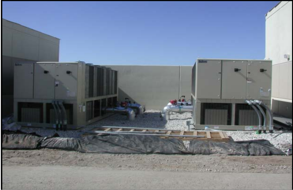
Figure 6.4 A high-energy efficiency HVAC system installed at Watergrass.
