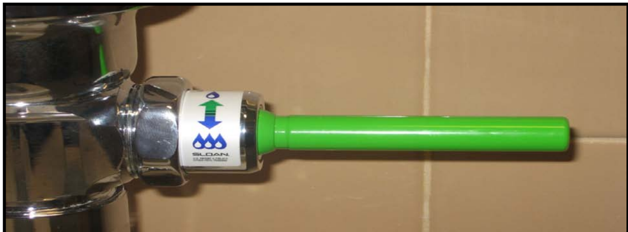
Figure 6.3 A dual flush valve was installed in the restrooms for water use reduction.
